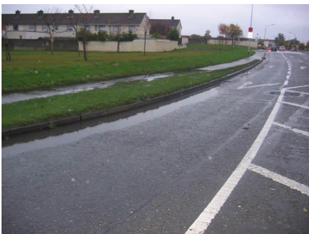
Localised ponding caused by low spot or blocked gully.
