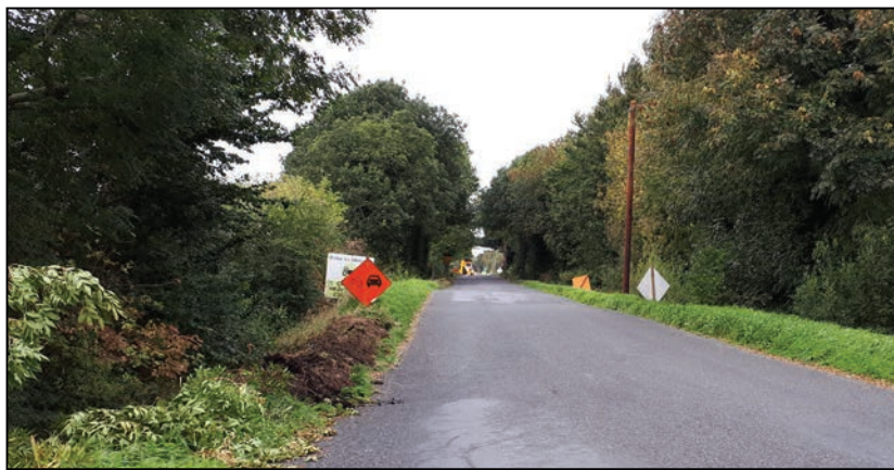
Figure 3.2 - Example of Undulations & Edge Failure on Road over Peat
